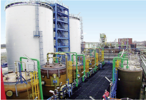
Salt storage & Brine treatment, Dormagen, Germany
