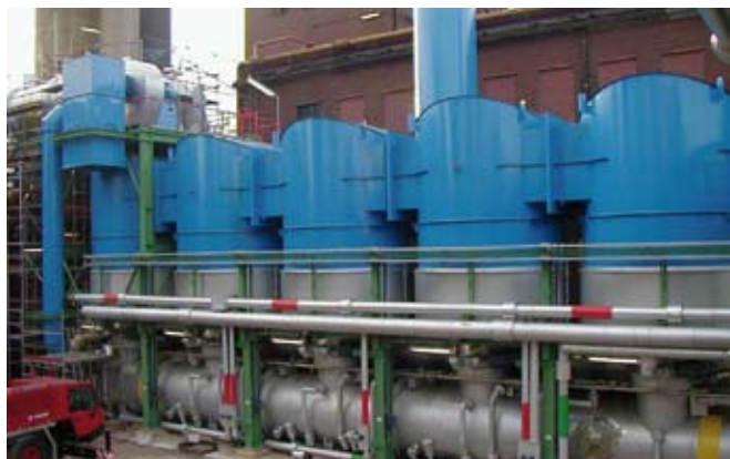
Thermal reactor for the PSA plant, Uerdingen, Germany
