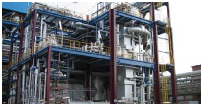
TAREX® Unit of TAD plant in Dormagen, Germany
