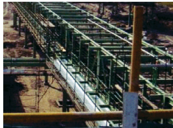
Pipe bridges play a central role in the supply of industrial plants
