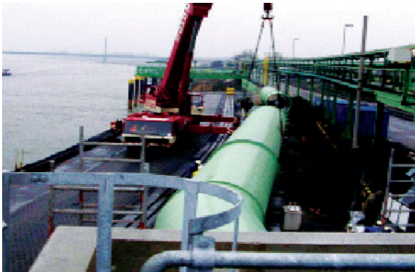
High-water pumping station with transfer piping (DN 2400)
