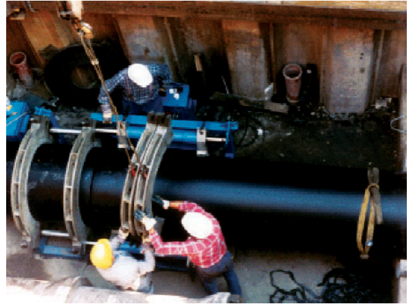
HDPE pipe connection (DN 1000)
