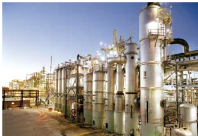
Production Facility in Baytown, TX USA
