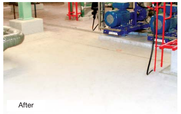
Following the demolition and replacement of several thousand square meters of defective basement flooring (above), the floor is again leaktight (below); during the reconstruction work the plant was able to continue working.
