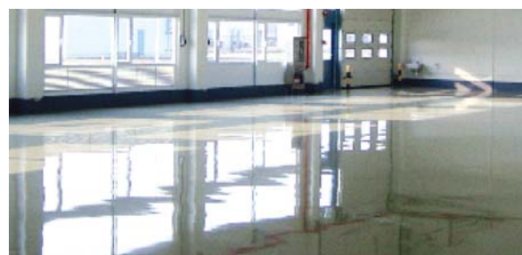
Flooring for storage area with a jointless coating
