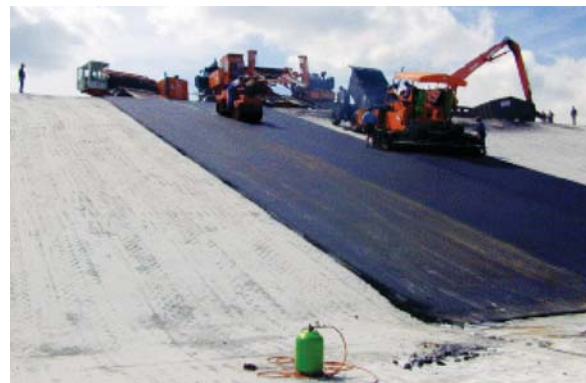
Installation of an asphalt surface sealing layer to secure a contaminated site
