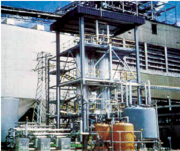
LOPROX®, plant, La Felguera, Spain
