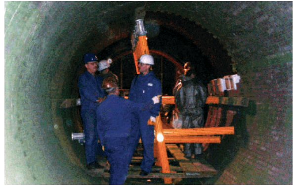
Refractory lining for the rotary kiln at a hazardous waste incineration plant
