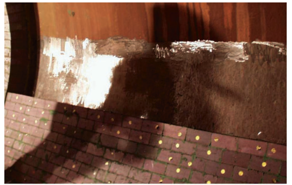
Refractory lining for a rotary kiln
